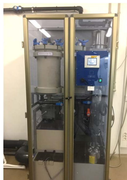
Water treatment unit
