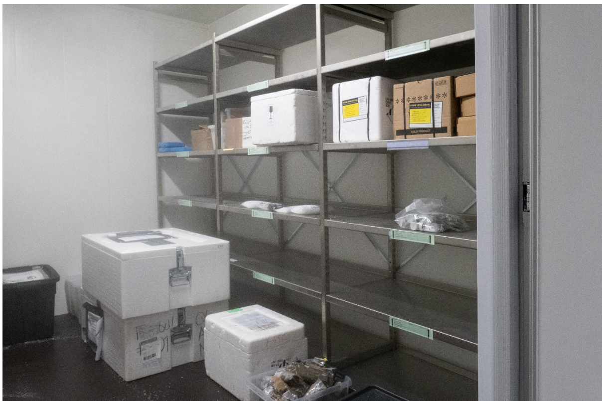
Freezer room (photo: Kai Mortensen)
